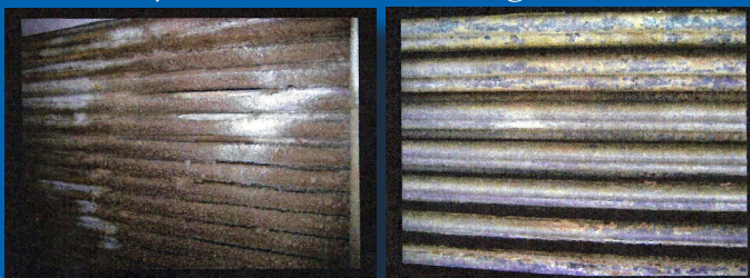
Reduction of interior scaling in cooling tower after just a few weeks of using Soft Wave
