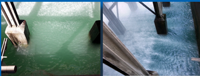
Change in cooling tower water after just a few weeks of using Soft Wave
